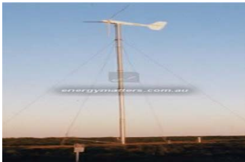
Figure 13. The 20 KW wind turbine. From [9]
